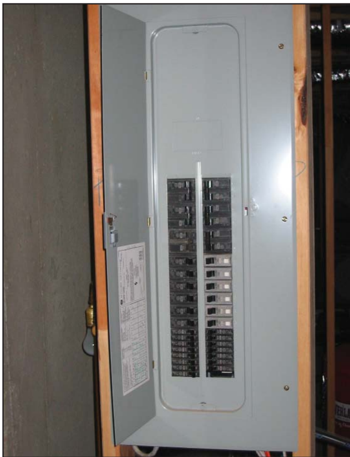
Figure 11.14. 200-Amp Service Box
