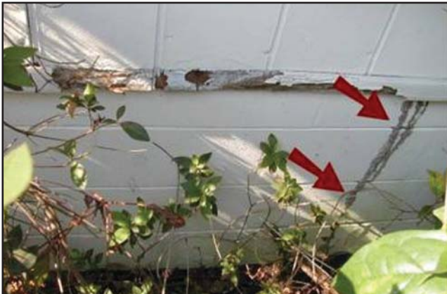
Figure 4.18. Termite Tube Extending from Ground to Wall [Red Arrows] [13]
