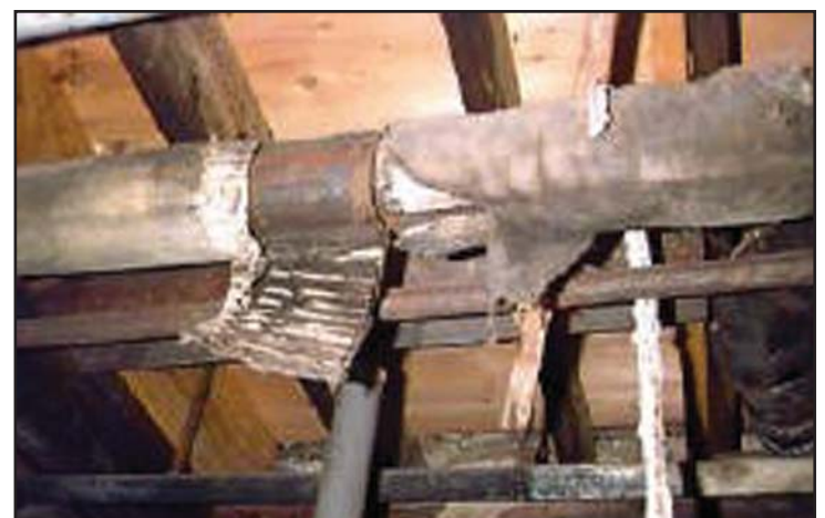
Figure 12.6. Heating Ducts Covered With Asbestos Insulation
