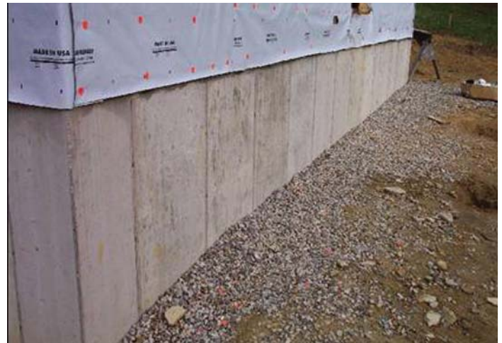
E. Gravel fill is placed outside the finished poured concrete foundation. This ensures that moisture does not stand around the foundation for any time. The moisture is routed to the footing drain for fast dispersal.
