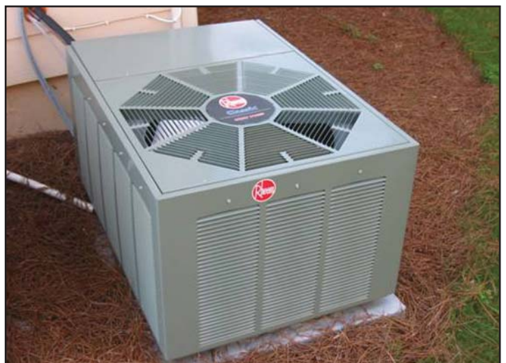
Figure 12.21. External Air-conditioning Condenser Unit
